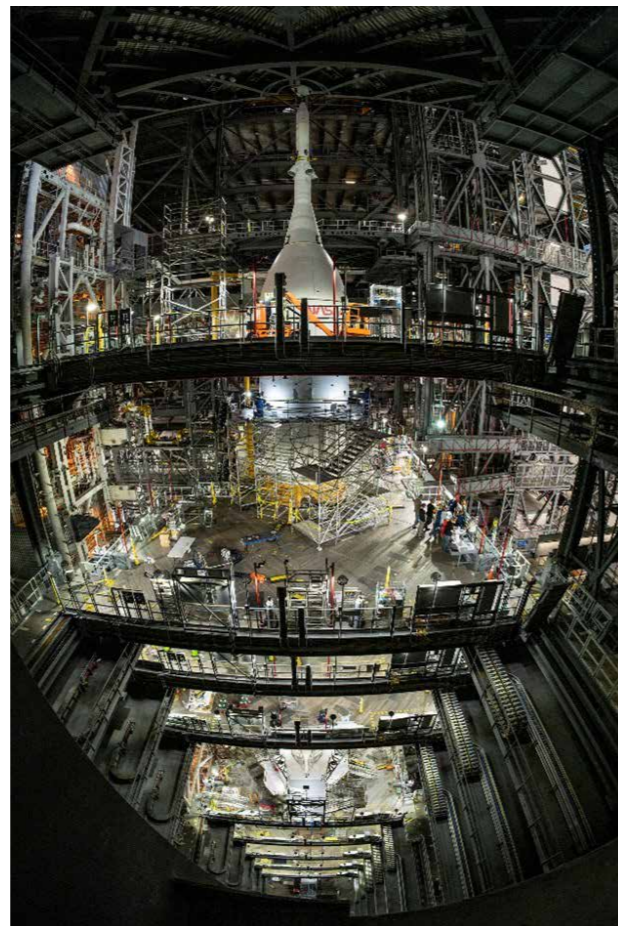
A view of the fully stacked Orion and SLS in the Vehicle Assembly Building
